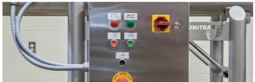
Control panel - NEMA 4X
